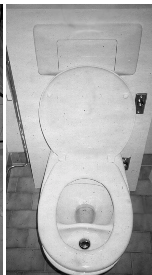
Fig. 34 - Urine collection area adequate
